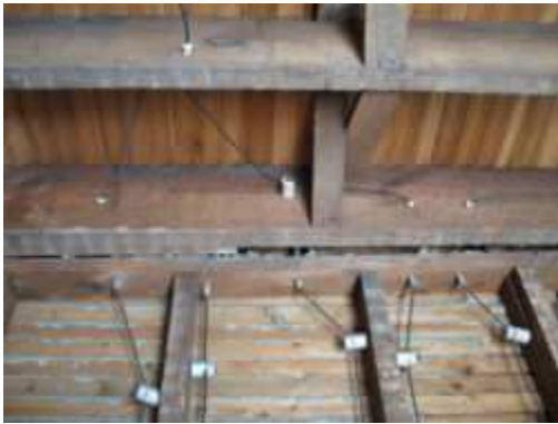
Example of Knob and Tube Wiring from a 1930's house.
